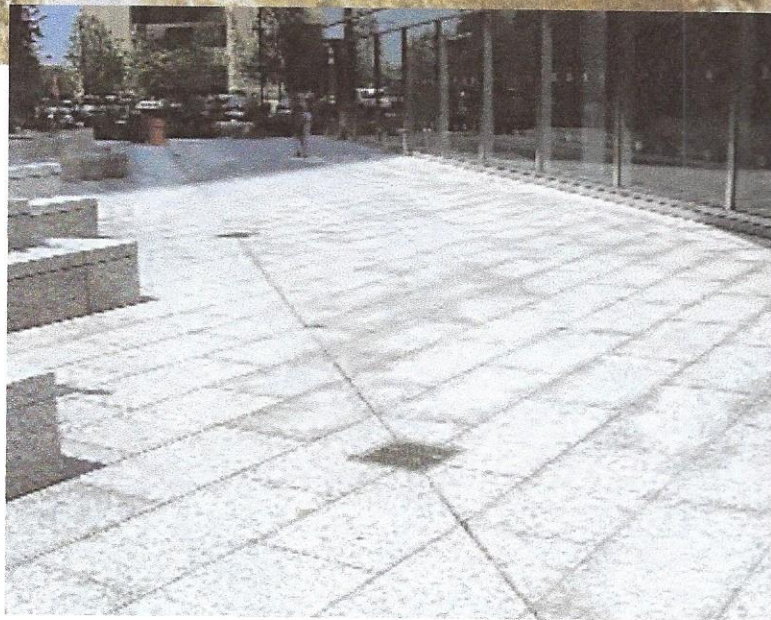
Moisture damage on exterior floor slabs.
